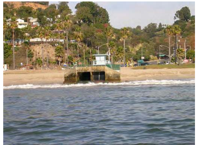
Los Angeles storm drain entering the ocean. (Photo credit: Phyllis Grifman, USC Sea Grant)
